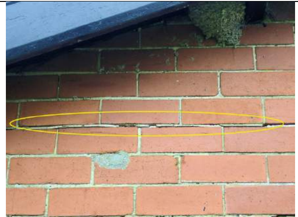
Fig 13: Corrosion induced expansion cracking to the rear gable wall.
