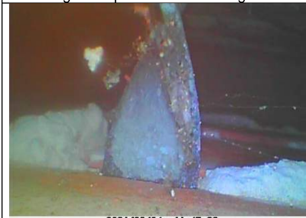
Fig 3: Early stages of red rust corrosion – left wall.
