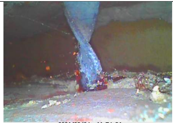
Fig 8: Advanced red rust corrosion – rear gable.
