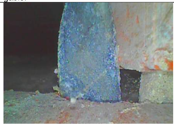
Fig 10: Early stages of corrosion – right wall.
