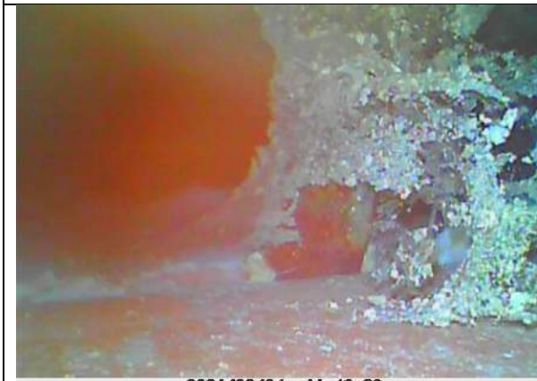
Fig 5: Advanced stages of red rust corrosion - left wall.
