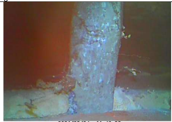
Fig 4: Early stages of corrosion – left wall.
