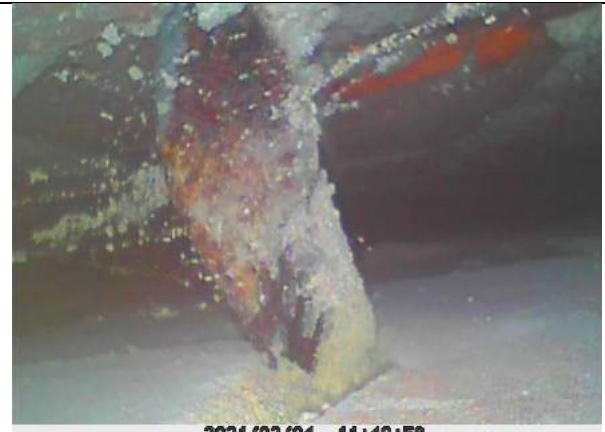
Fig 2: Severely corroding tie to the front gable.
